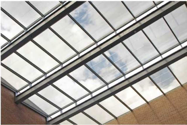
FIGURE 12.15 Skylight with semitransparent a-Si PV cells. Courtesy of Onyx Solar llc©.
