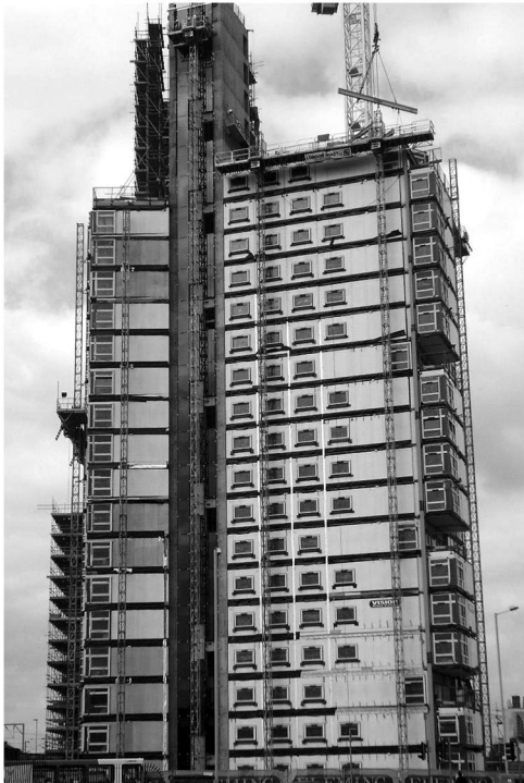
Fig. 8. 25-story modular building in Wolverhampton, England, during construction (image by R. M. Lawson)
